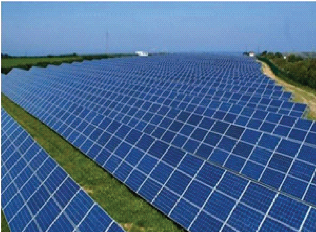
Fig. 1.2.1 Solar PV plant
