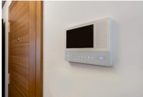
Fig. 1.1.12: Proximity security system
