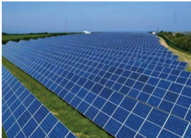
Fig. 1.2.1 Solar PV plant
