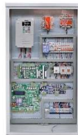
Fig. 1.1.4: VSD control panel
