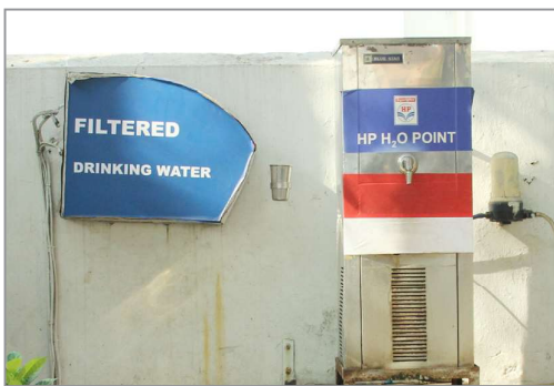
Fig. 2.1.12. Drinking water facilities
